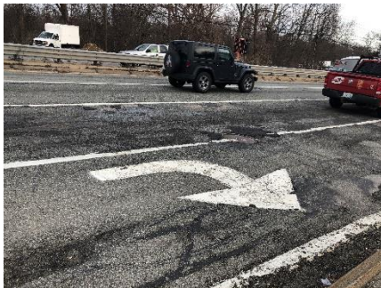
Figure 4 -- Delaminated Pavement on RI-146 at Sayles Hill Road
